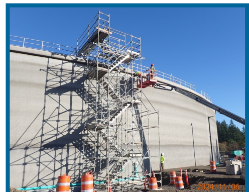
Reservoir roof lightning protection ground wires installed on the exterior walls
