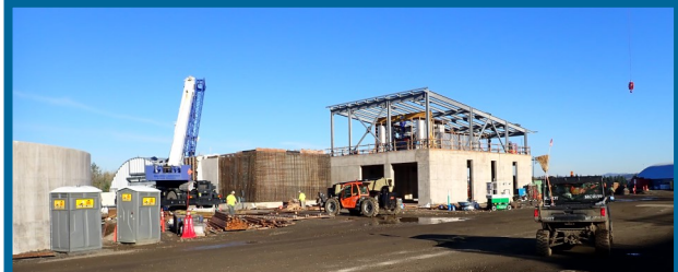
Dewatering area, which includes (from left to right) a thickener, formwork for a storage tank, and the dewatering building with structural steel and mechanical devices on the second floor
