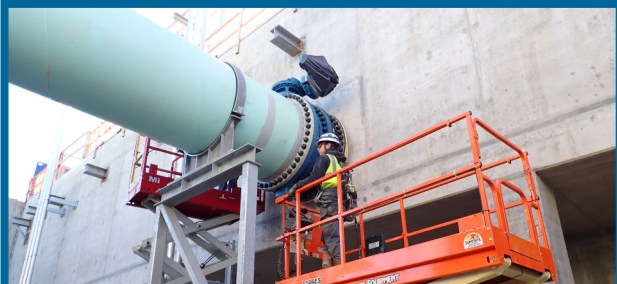
48-inch pipeline that conveys water from the ballasted flocculation process to the ozone contactors
