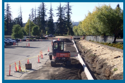
Mini excavator grading rock in a parking lot to prepare for paving
