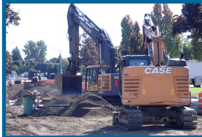
Excavator being used to prepare for temporary paving on SW 95th Ave.
