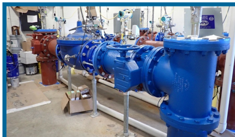
MPE_1.2: Valve testing at Pressure and Flow Control Facility
