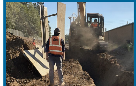
Installing shoring for drainage piping on access road north of NE Cherry Drive
