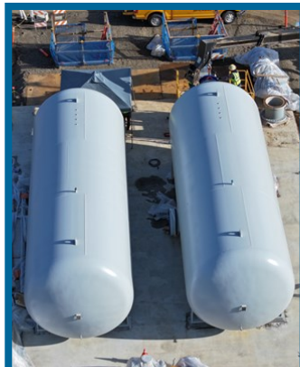
Surge control tanks
