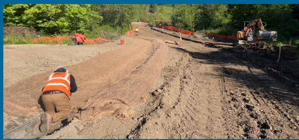
Jute matting installation at a drainage swale in Orenco Woods Nature Park
