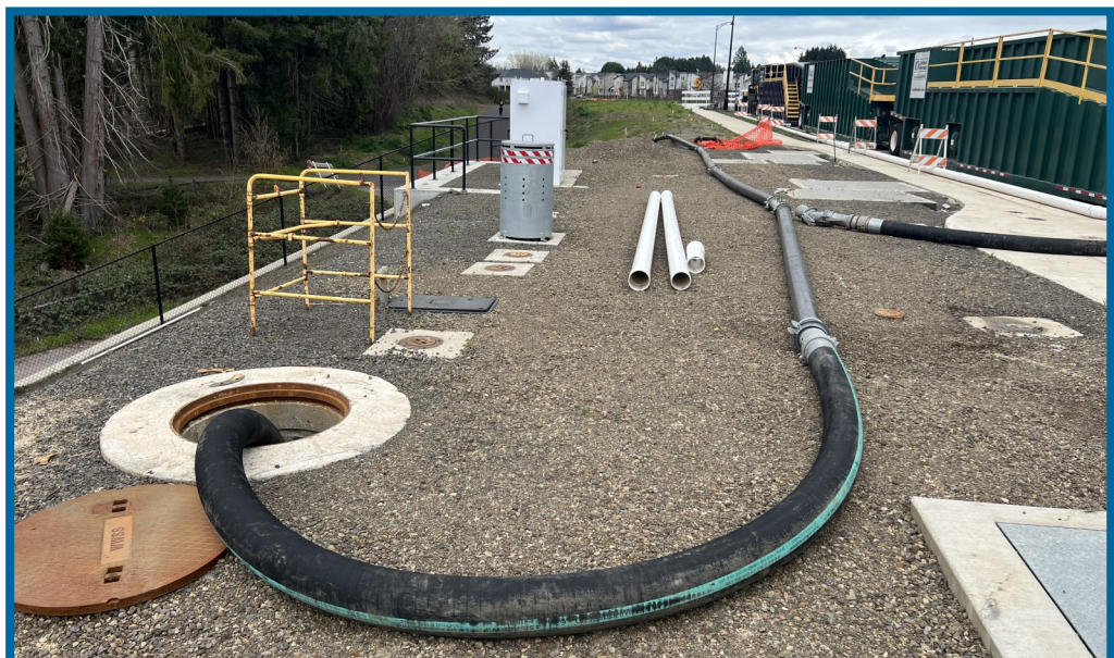
Temporary piping setup during chlorination and flushing of the 48-inch and 66-inch water pipelines
