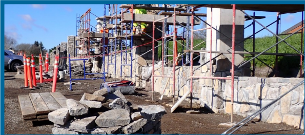
Castle Masonry installing stone veneer on the southern section of the Raw Water Facility's perimeter fence
