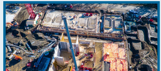
Aerial view of construction of the flash mixing and ballasted flocculation areas (bottom) and the chemical storage area (top)
