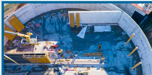
Aerial view of construction of the 10-million-gallon finished water storage tank (clearwell)
