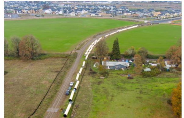
The South Hillsboro Area Pipeline Segment is approximately four miles in length.
