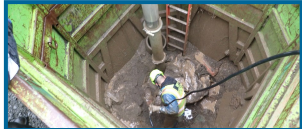
Vac truck excavation of man way flange (prework for PLM_5.2 and PLM_5.3 tie-in)
