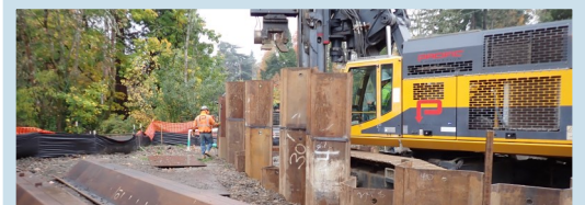
MPE_1.2: Contractor driving z-piles for jacking pit shoring in advance of trenchless pipeline installation
