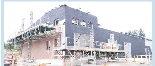
RWF_1.0: Electrical building concrete masonry unit (CMU) with brick veneer wall construction
