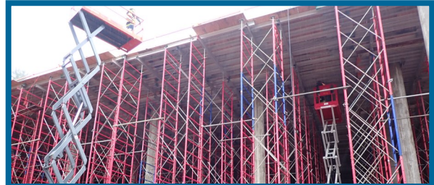
Scaffolding used to support the decking for the roof of the reservoir tank
