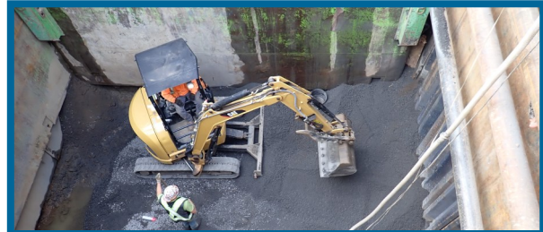
Construction crew preparing the bore pit at 124th Avenue and Tualatin Sherwood Road.
