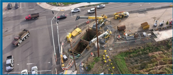
Aerial view of the trenchless pipe installation operation at 124th Avenue and Tualatin Sherwood Road.
