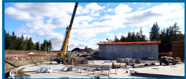
Completed foundation slab at the clearwell (with finished water pump station wet well in background)
