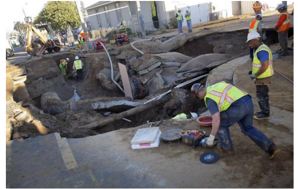
Crews assess infrastructure damaged from an earthquake in California. Advanced construction techniques used for the Willamette Water Supply will limit damage and help to maintain critical services to water customers during emergencies. Photo: Carlos Avila Gonzalez, The San Francisco Chronicle
