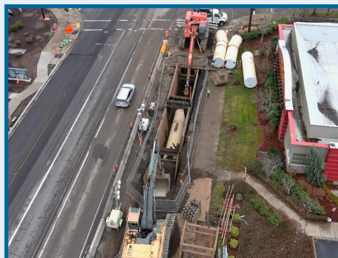
January 2023: Installation of 66-inch pipe along Tualatin-Sherwood Road near Langer Farms Parkway.
