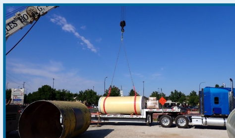
August 2022: Delivery of 66-inch carrier pipe for the 99W trenchless crossing along Tualatin-Sherwood Road.
