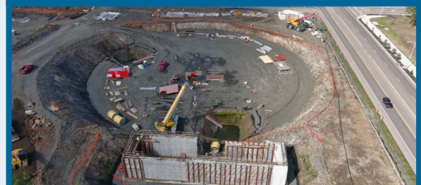
Excavation for the 10-million-gallon circular finished water storage tank and lower walls at the finished water pump station
