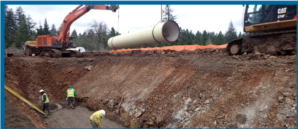
Pipe bedding, final grading, and pipe mobilization to trench along Grabhorn Road
