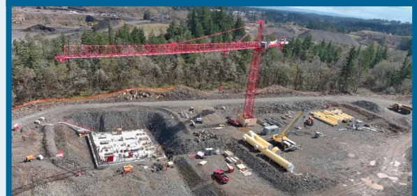
UV area lower slab (left), tower crane (middle), and stored large-diameter pipe (right)
