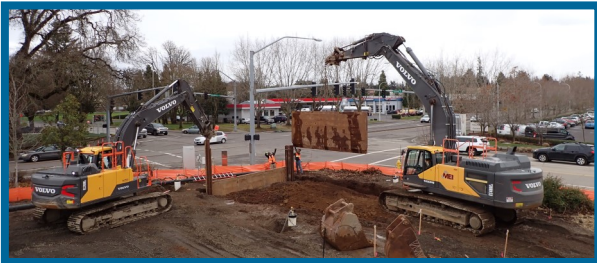
Contractor installing slide rail shoring for a trenchless crossing jacking shaft on the south side of Wilsonville Road
