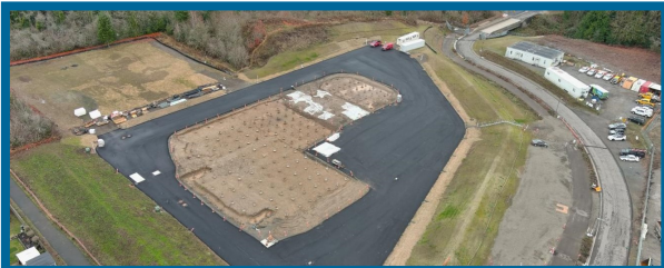
Upper Site: Electrical building excavated to subgrade and pile tops exposed and cleaned in preparation for under-slab conduits, aggregate base rock, and building slab reinforcing.
