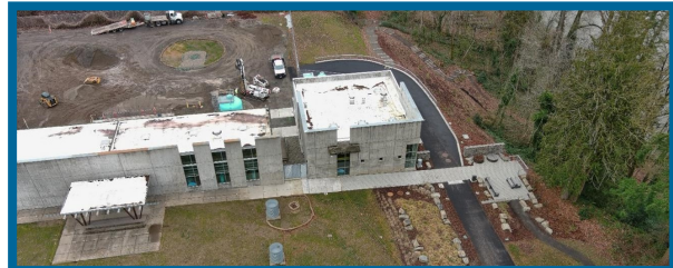
Raw Water Pump Station & Lower Site Area: Completed permeable asphalt, drainage improvements, overlook area, pedestrian paths, and landscaping.
