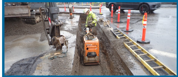
Compaction of 12-inch City of Beaverton waterline trench in Beaverton Hillsdale Highway
