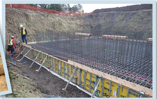
PLM_4.3: Creating walls for the Tualatin River trenchless crossing via North Shaft overlapping installations
