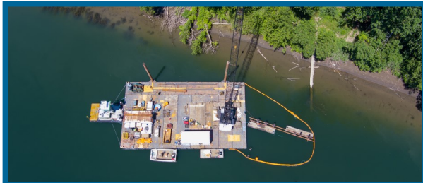
Barge and crane for in-water pile driving operation at fish screen protection fence
