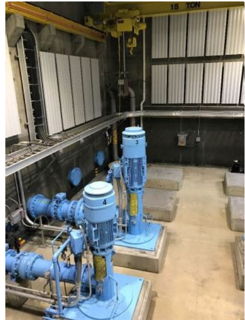
Existing WRWTP pump station
