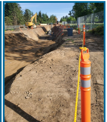
A safe distance from the edge of the trench is clearly marked for workers needing access above the trench.
