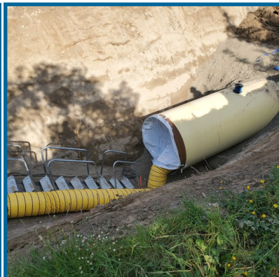
Proper ventilation is necessary for welders working inside 66-inch diameter pipe. Forced air is pumped through the pipe and air monitoring is performed.
