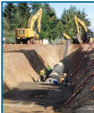
While installing 66-inch diameter pipe, safe trench access and egress is essential for workers in emergency situations.
