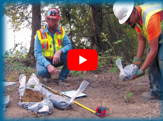
Jason Bock, Senior Engineer with GRI, studies soil samples for the Arrowhead Creek pipeline crossing in Wilsonville.
