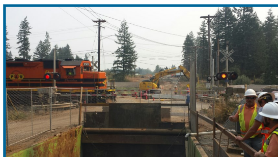
Installation of steel casing pipe at railroad tracks on SW Tonquin Rd.
