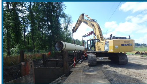
Installation of last 66-inch diameter piece of pipe for the Kinsman Project
