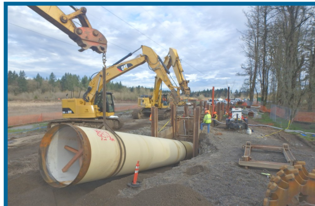
Crews from Emery & Sons Construction place pipe into a trench on the Kinsman Road Partnership Project ( watch video )
