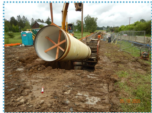
The 66-inch pipeline is being installed on Scholls Ferry Road, Tile Flat Road and Roy Rogers Road.
