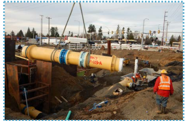
Almost 2,500 feet of drinking water pipeline has been installed in the South Hillsboro area.
