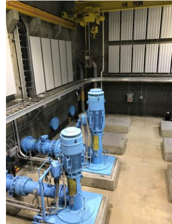
Existing WRWTP pump station
