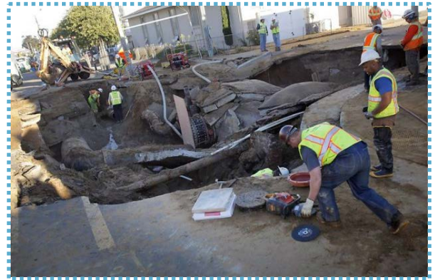
Crews assess infrastructure damaged from an earthquake in California. Advanced construction techniques used for the Willamette Water Supply will limit damage and help to maintain critical services to water customers during emergencies. Photo: Carlos Avila Gonzalez, The San Francisco Chronicle
