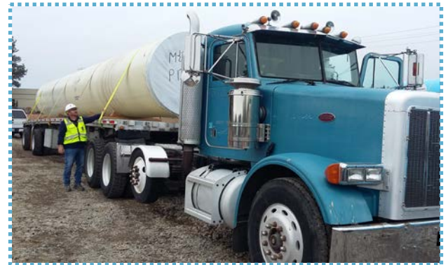
A 66-inch diameter piece of pipe sits on a truck waiting to be unloaded and installed at a Willamette Water Supply System construction site.
