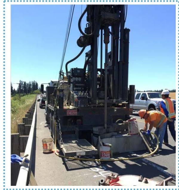
A drill rig will soon be sampling soils in the Willamette River Water Treatment Plant Park
