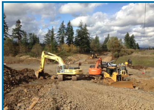
Location of new 124th Ave. and Tonquin Rd. intersection as part of the 124th Avenue Partnership Project
